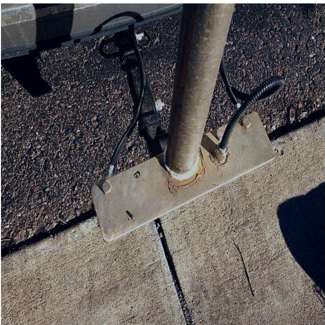
Top Of Antenna Mount (Looking Down)
